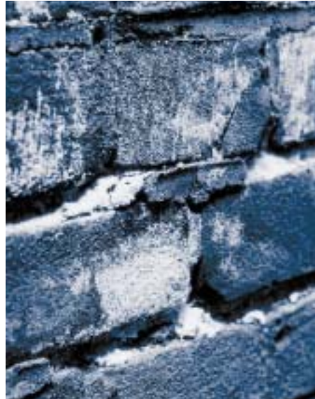
Figure 1 Push out of pointing, provoked by salt crystallisation
