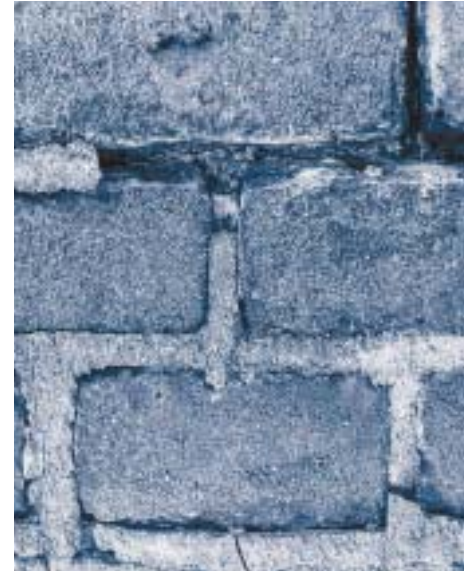
Figure 2 Push out of pointing, provoked by frost action. The choice of the pointing mortar composition may determine the extent of the damage
