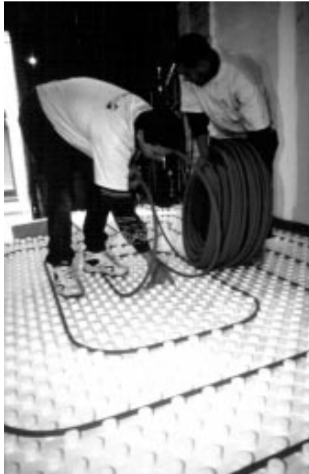
Symphonie software can help optimise the design of heated floor systems, among others
