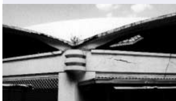
Algeciras Market (below) – Detail of the deterioration of the reinforced concrete
