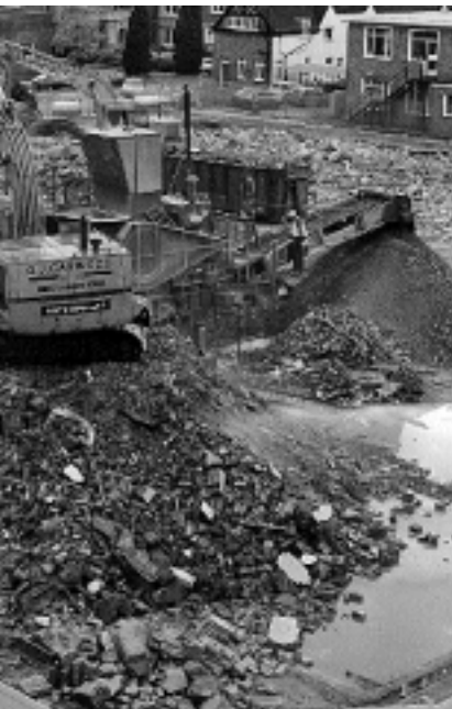
Used on site to provide hardcore for the tilt at the home of BRE in the UK
