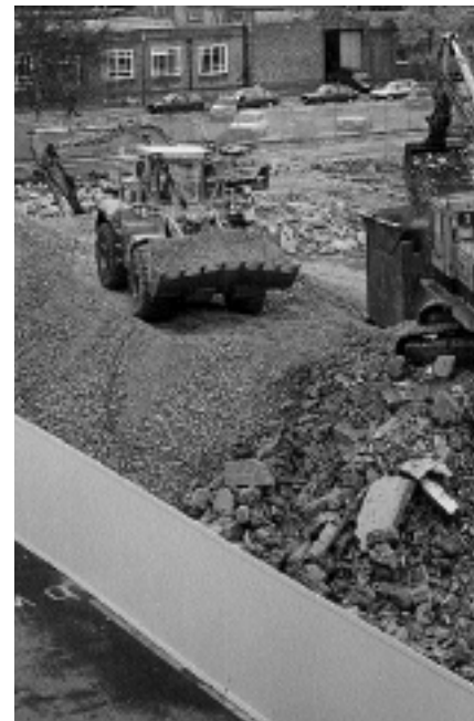
Demolition waste from old buildings is crushed. Energy Efficient Office of the future now built.
